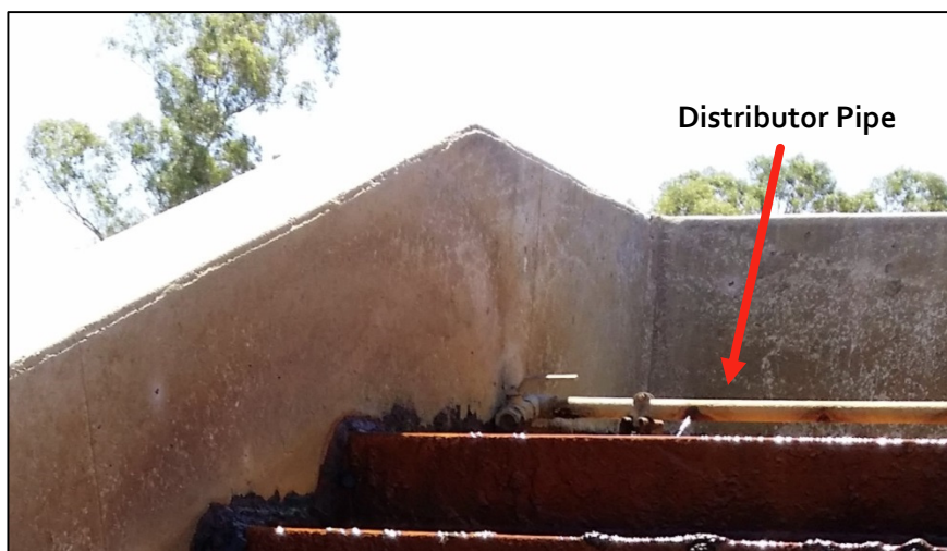
Figure 4-3: Distributor Pipe at Top of Aerator for \text{KMnO}_4 and ACH Dosing
