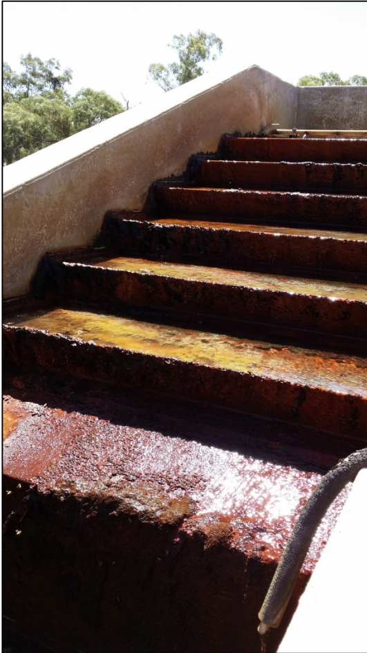
Figure 4-1: Step Aerator (during Down Time)
