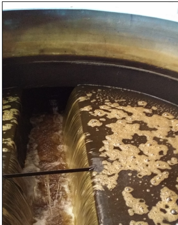
Figure 4-12: Filter 1 during Backwash Showing Manganese Contaminated Wastewater
