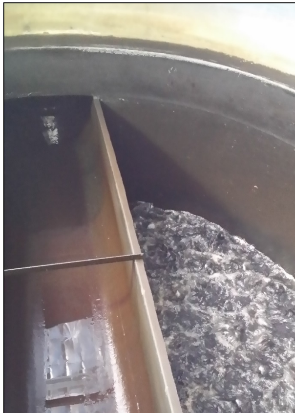
Figure 4-11: Inside Filter 1 during Combined Air and Water Backwash
