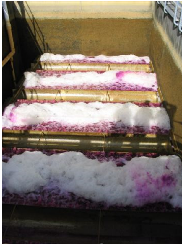
Figure 7-1: Filter Media being Coated with Manganese Oxide
